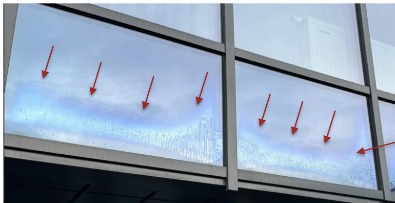
Areas of damage to the glass coating
